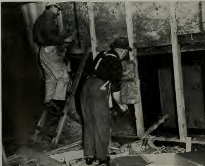
Fitting the Fiberglas insulation between the studs of the bulkhead separating the hold and the combined galley and forecabin.
